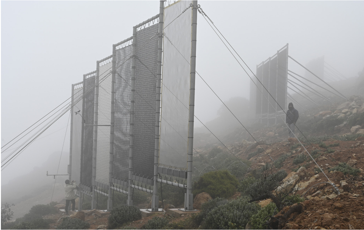
Figure 1 Fog water collection systems (Credit: Aqualonis).
